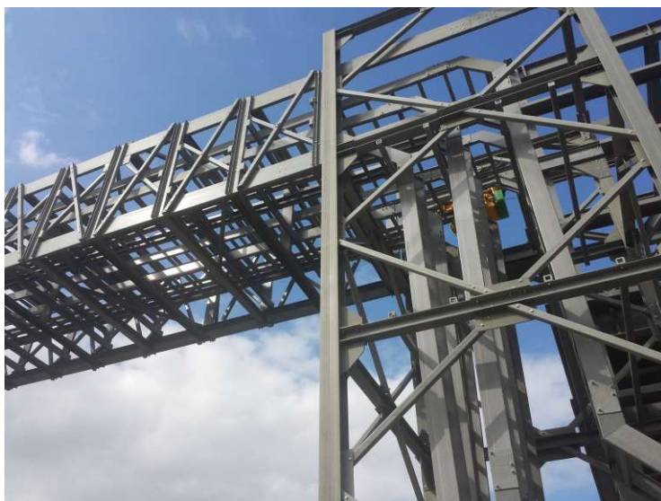
Cable Rack - Porto do Sudeste
